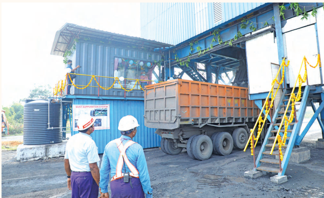
Dust Suppression System arranged at Pre Weigh Bin Truck Loading System in Kistaram OC, KGM Area
