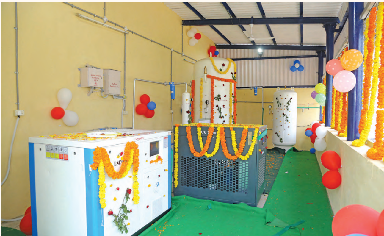
One of the 5 Oxygen Generation Plants established in SCCL area Hospitals (Bhupalapalli Area)
